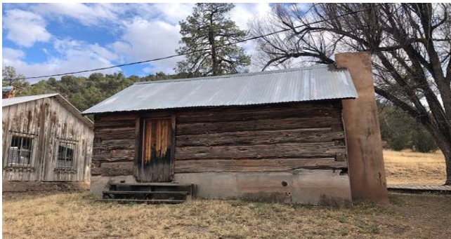
The Post Office cabin, one of the few original structures remaining today. Photo Charles Doran.
