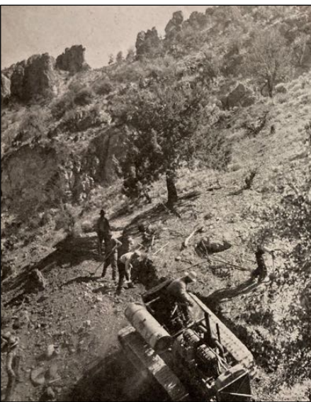
A Caterpillar tractor working on the road between Hillsboro and Kingston in 1929, "sticking to the side of the hill like a mountain goat and doing its work where the going is toughest." The photo was included as part of an ad in the New Mexico Highway Journal , July 1929.
