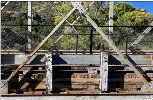
Detail of the bridge, showing the steel trusses and wooden decking under the roadway. Photo Joe Britton.
