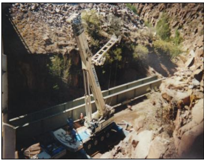
Construction of a new bridge at the box canyon in 1995 to replace the original 1927 truss bridge. Photo Phyllis Glines.
