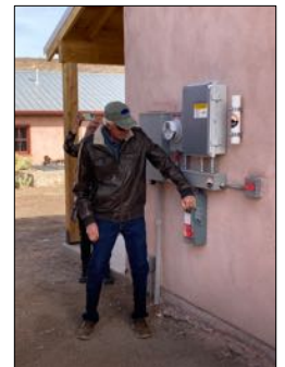
"Flipping the switch" on February 1 to activate the new Coach House solar panels.
