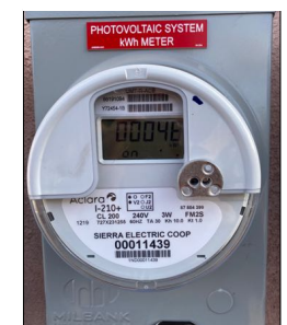
Meter showing the electricity generated by the solar panels, producing enough to power the entire Black Range Museum.
